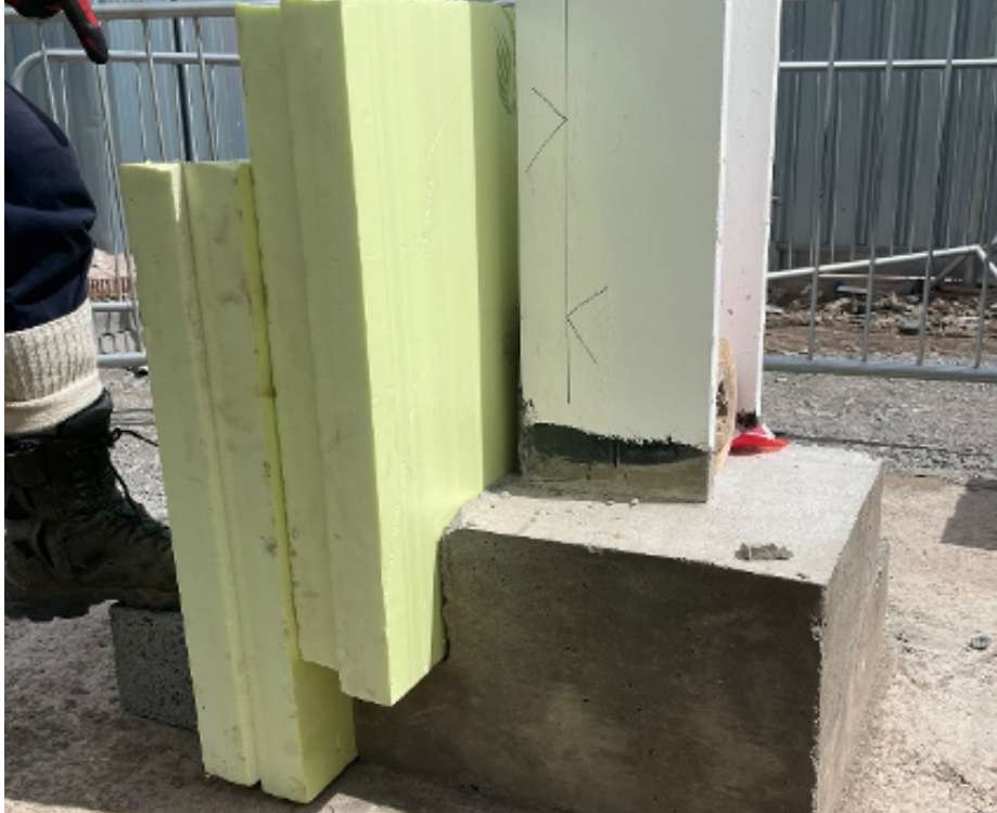
Quality led sub-structure details at Faifley Campus as a result of sub-contractor early engagement and testing to develop solutions.
