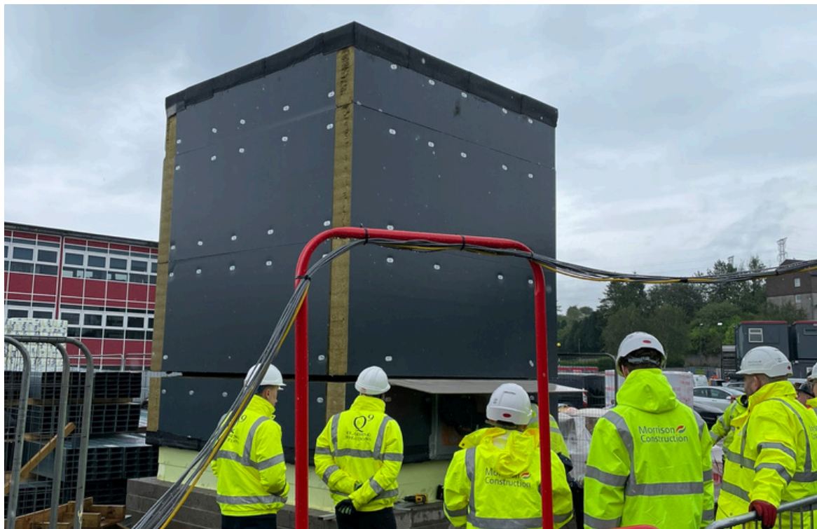
Morrison Construction using test rigs on site at Faifley Campus to test key junctions with supply chain ahead of site install
