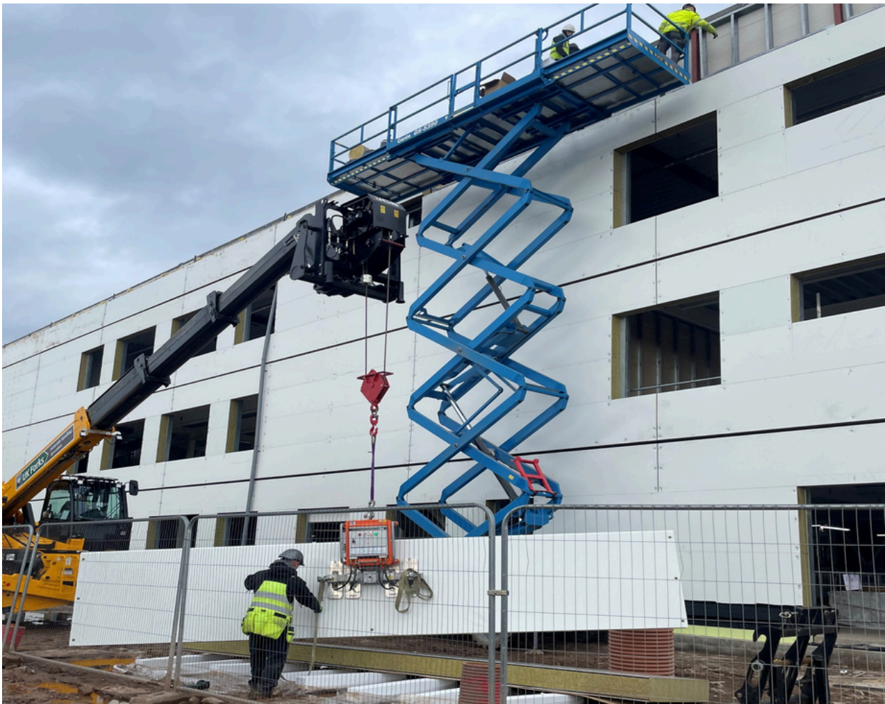
Installation of composite panels at Faifley Campus- Morrison Construction developed a DfMA solution with the supply that started with the test rig at BE-ST
