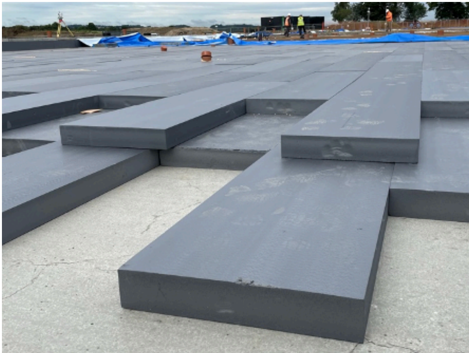
Ground slab solution at Maybury Primary School: Morrison Construction worked with their groundworker to introduce a concrete blinding to create a flat surface for insulation slabs.
