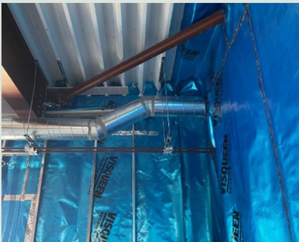
Image highlighting complexities of achieving internal airtightness lines highlighting the range of interfaces that it is required to seal around/ against.
